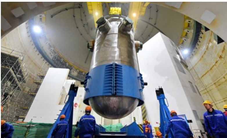
TNR instalovaná na Fuqing 5 (Image: China Nuclear Engineering & Construction)
